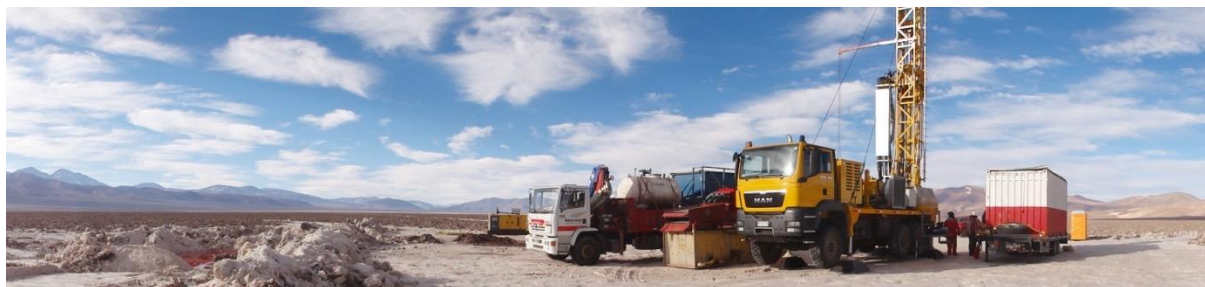
Figure 1: Hellema Holland Praxla rig drilling the pump test well in Cocina tenement
