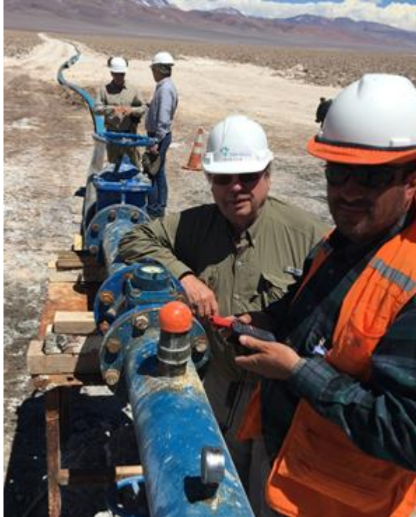
Figure 4: P4 pump test pipeline
